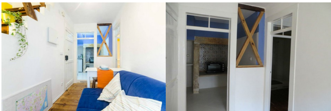
Renovation of an old house in Lisbon, CAS (Paulo Carneiro & Alina Jerónimo)
