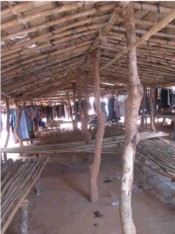
Bamboo and wooden structure in informal market in Manica, Mozambique. Photo by Paulo Carneiro
